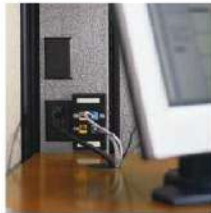
Above Work Surface Electrical
